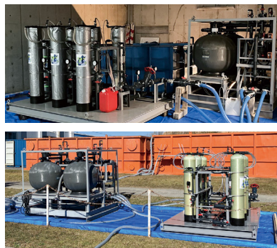
Water treatment system installed
